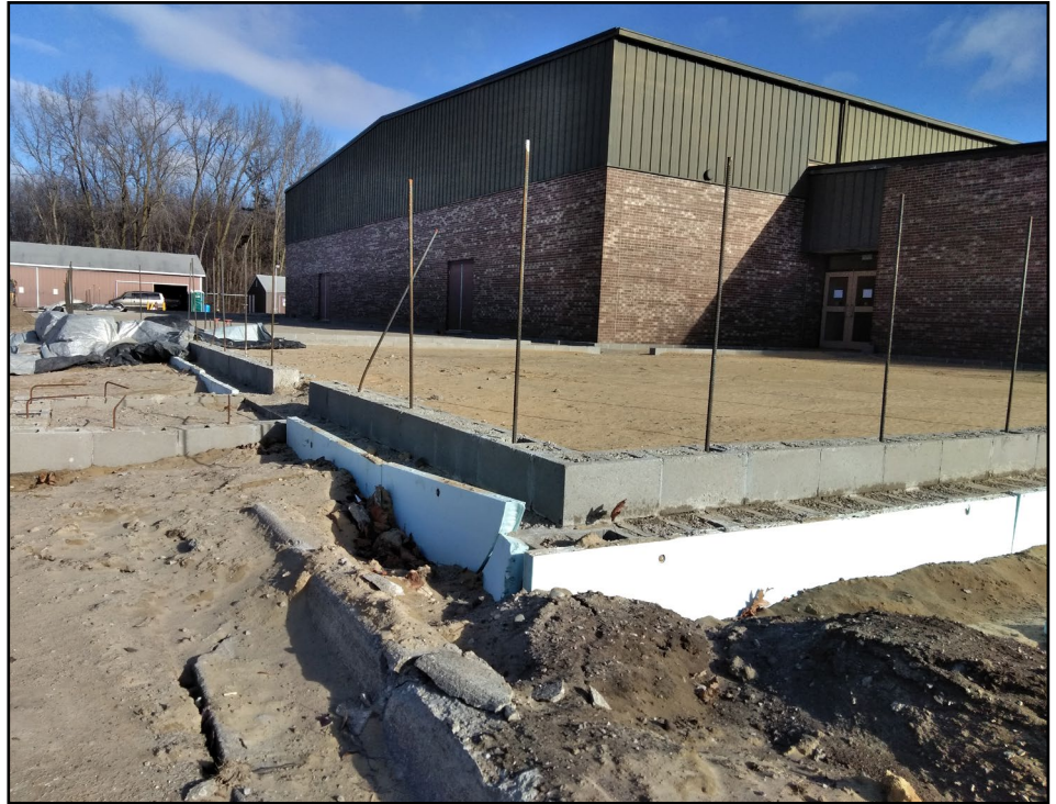
Footings have been poured and the ground leveled in anticipation of wall construction on the west side of campus.
